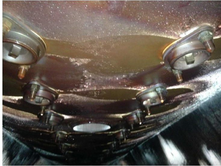
Figure 1: Deaerator dome and spray nozzles with water droplet accumulation
